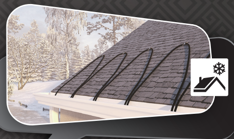
Roof and gutter de-icing system.
